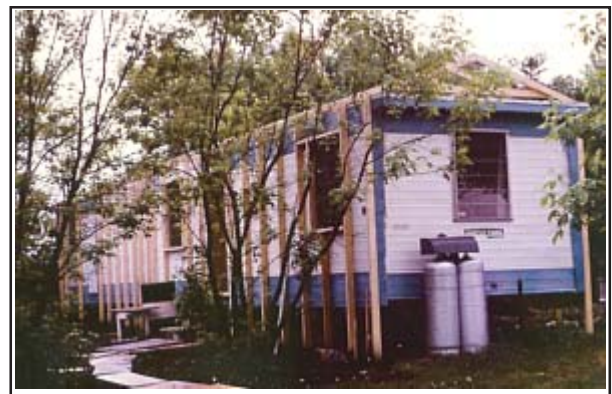
The mobile home undergoing remodeling in order to serve as housing for Kamsack missionary couples
