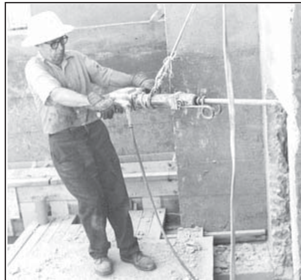
Cutting through the original basement wall to create an inside the basement access into the storage room.
